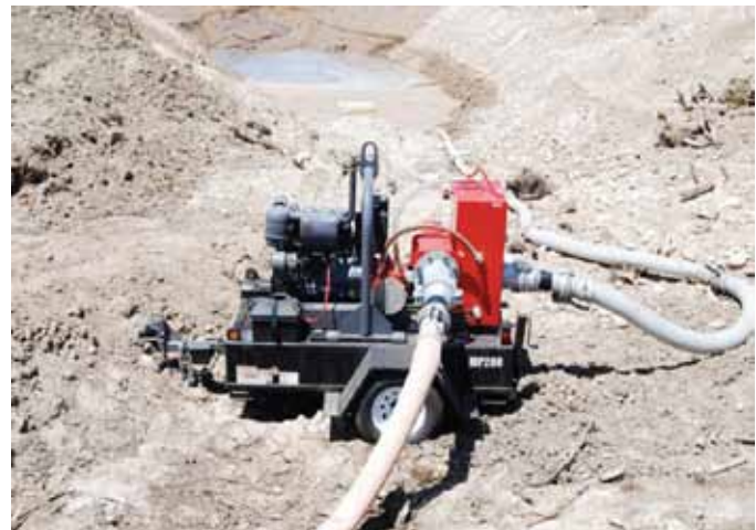
This 8" pump was reduced to 6" hose on a long term rental of construction site dewatering. It outperformed the 6" pump it replaced, and also used less fuel.
